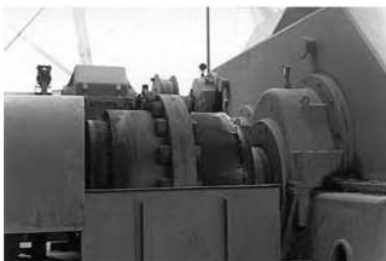
Cement kiln mill drive
